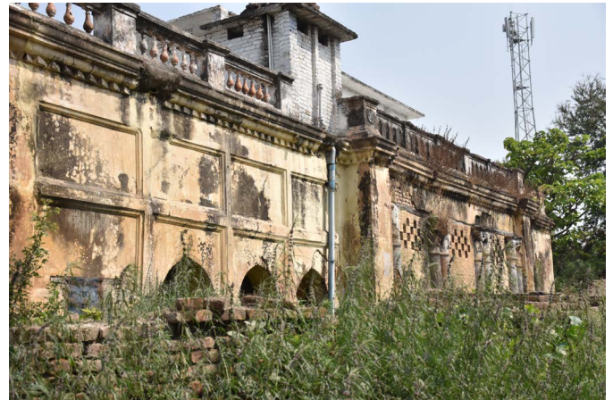
Figure 31 : Pappu Singh Residence, Bharatkand, Parbatta Source: Primary survey by AH Division, INTACH Team
