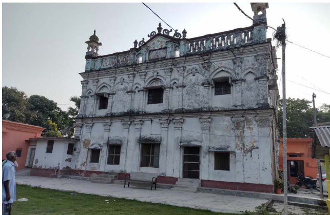
Figure 20 : Uchhla Estate Kothi, Bhandartal, Barari Source: Primary survey by AH Division, INTACH Team
