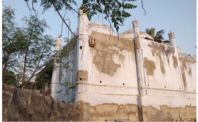
Figure 9 : Shahi Masjid, Medinipur, Manihari Source: Primary survey by AH Division, INTACH Team
